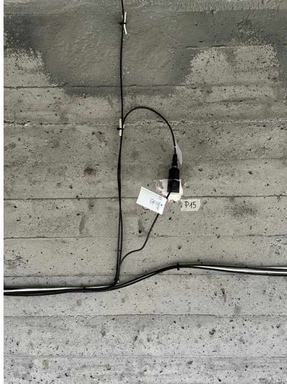
Fig. 48 Example of sensor placement under the bridge.
